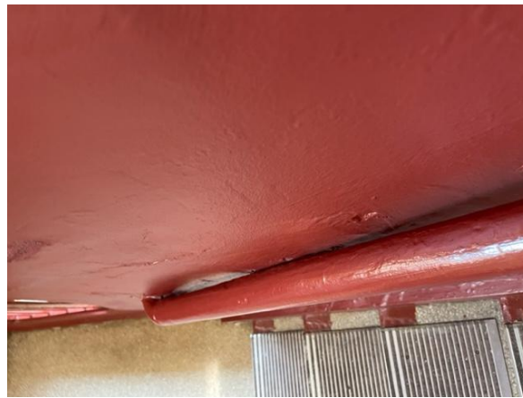
Figure 2: Bulging wall against handrail
